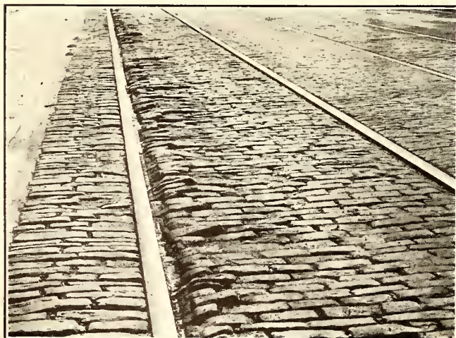
UNEVEN PAVING ALONG OUTER RAIL DUE TO ATTEMPT TO HAVE TRACK GRADE FOLLOW CROWN OF STREET
